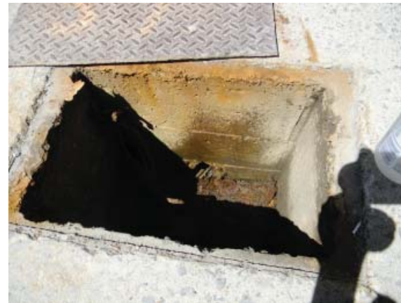
Photo 02: Transite electrical duct embedded in sidewalk
