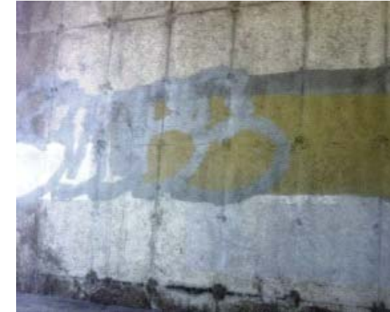
Photo 01: Paint on abutment walls (graffiti)
