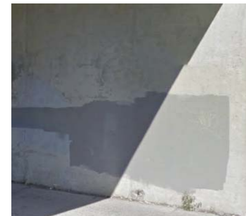
Photo 01: Paint on abutment walls
