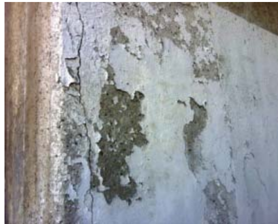
Photo 01: Paint on abutment walls
