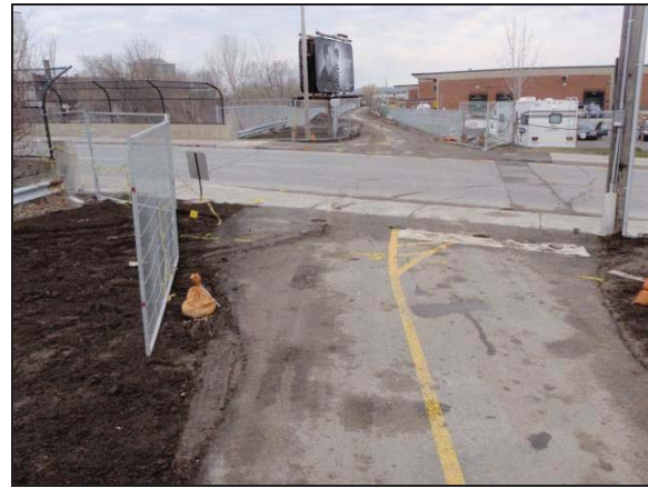
Plate 19: North view along east side of O-Train corridor showing recent recreational path construction.
