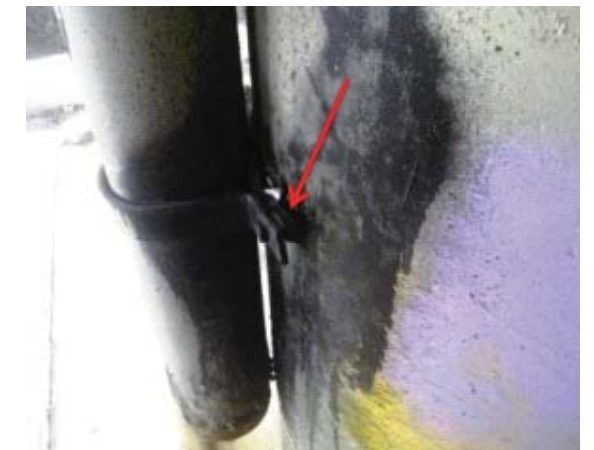
Photo 04: Drain Pipe Rubberised Isolator
