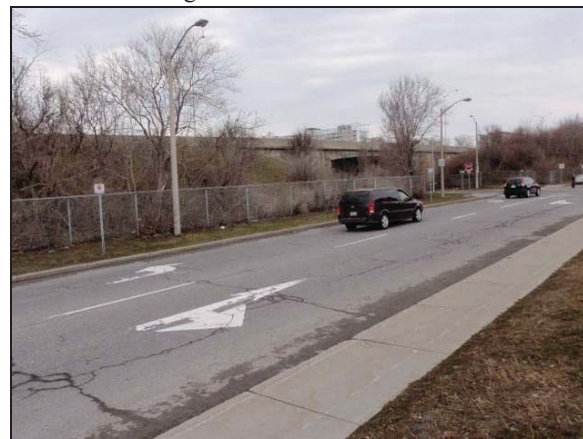
Plate 35: Northeast view of SW quadrant of Highway 417/Booth bridge along Orangeville Street.
