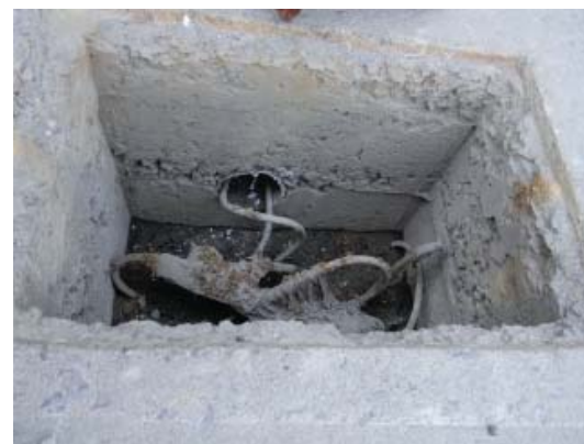
Photo 02: Transite electrical duct embedded in sidewalk
