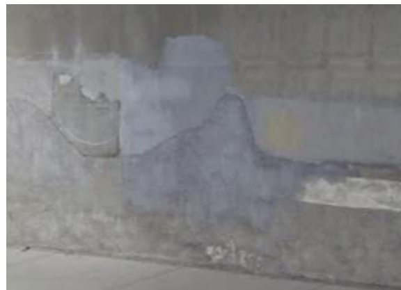
Photo 01: Paint on abutment walls
